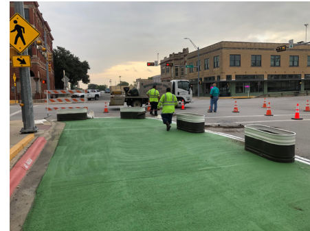
Public Works crews install planter boxes to the newly paved streetscapes located on West Second Street in downtown Taylor. Streetscape implementation is part of the 2015 Downtown Master Plan.
